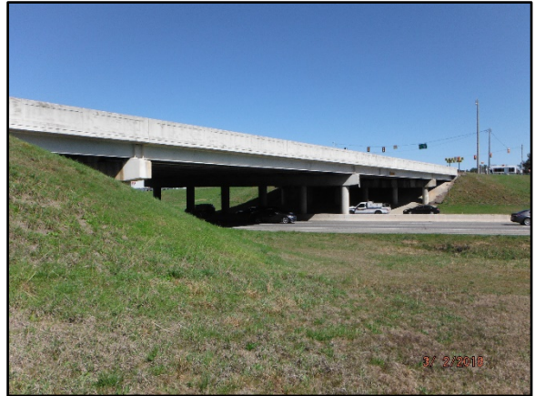
Photo 1 – View of the subject bridge, S-32-671 (Piney Grove Rd.) Bridge over I-26 looking up-station (Westward).
